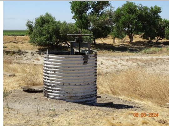
View of the gate operator on the right bank. (2024)
