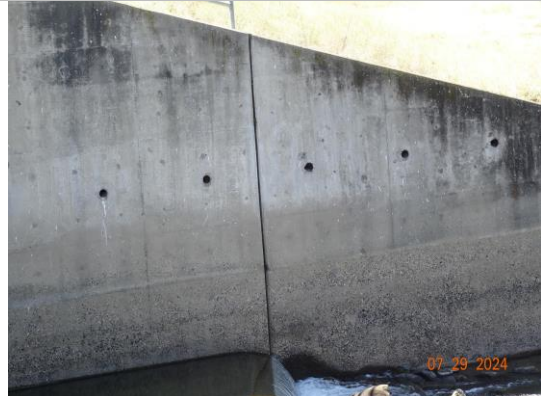
Felt in monolith joint on left wing wall has deteriorated. (2024)
