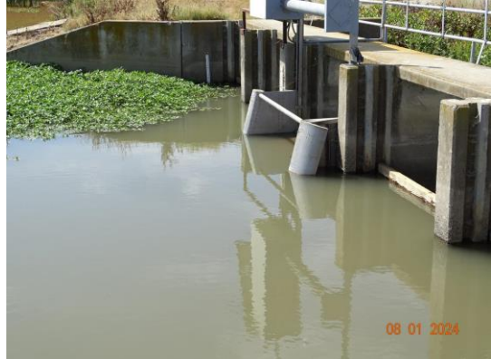
View of the upstream side of the structure from the right bank. (2024)
