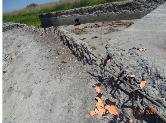
Damage to left wall of structure. (2021)
