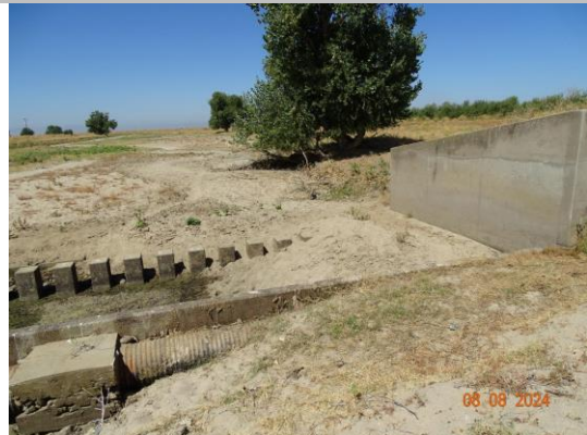
Sedimentation downstream along the right wall. (2024)
