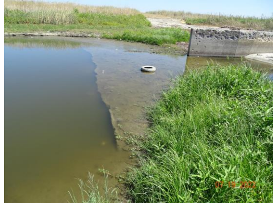
View of scouring on the downstream side of the structure. (2022)
