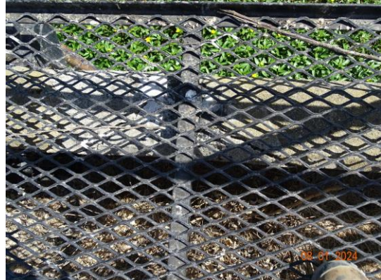
Small cracking on the headwall. (2024)
