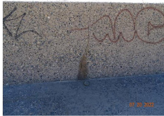
Small crack at head wall. (2022)
