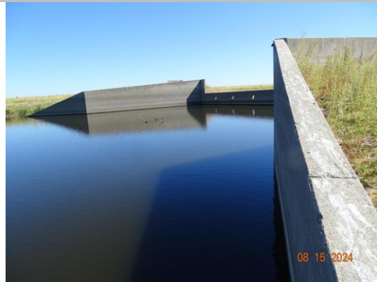
View of the downstream side of the structure from the left bank. (2024)
