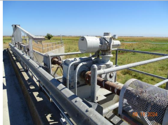
Typical view of electrical gates on upstream side of structure. (2024)
