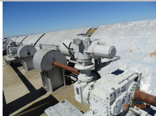
Typical view of the electric gate motors. (2024)
