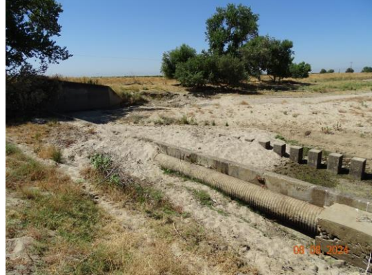
CMP that connect between culverts risers on left and right wing wall. (2024)
