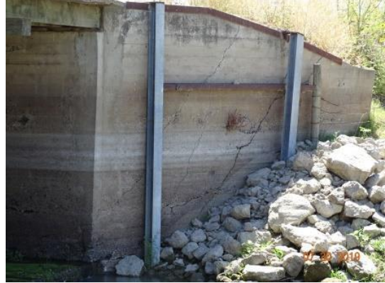
Looking at crack on left wing wall on downstream side of structure. (2019)
