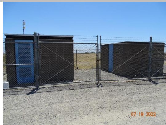
View of fencing around the electrical housing. (2022)
