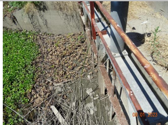
View of slide gate with sedimentation. (2023)
