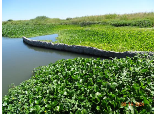
Damage to the right wall of the structure. (2024)
