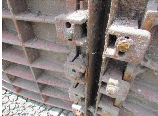
Looking at corrosion on slide gates on upstream side of structure. (2015)
