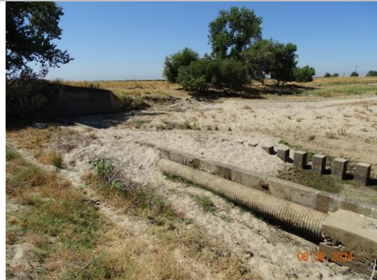
Sedimentation downstream along the left wall. (2024)
