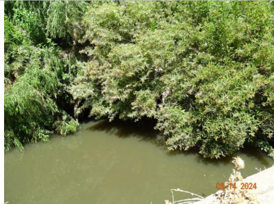
Trees growing over the downstream side of the structure. (2024)
