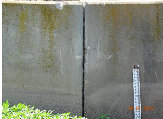
Deteriorating joint on the left headwall. (2024)
