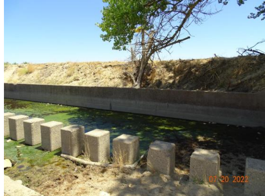
View of unauthorized earthen dam from downstream channel. (2022)
