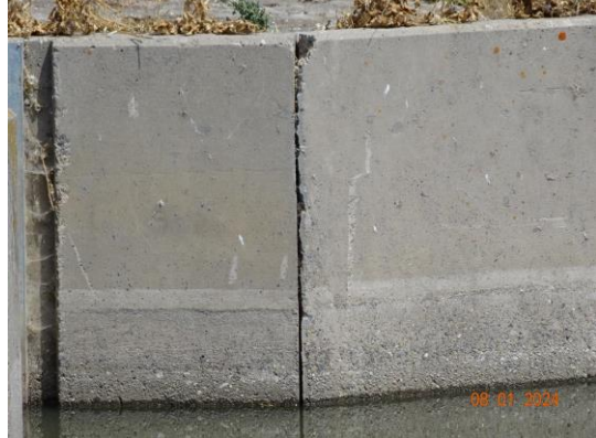
Deteriorated joint on the right headwall. (2024)
