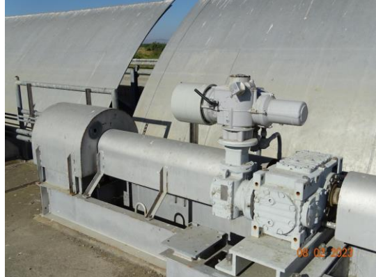
View of the electric gate operators. (2023)
