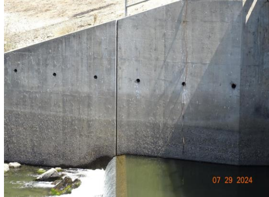
Felt in monolith joint on right wing wall has deteriorated. (2024)
