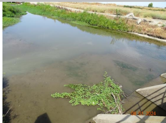
Erosion of the downstream revetment. (2024)
