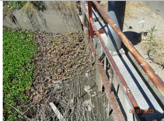
Sedimentation built up above slide gate. (2023)
