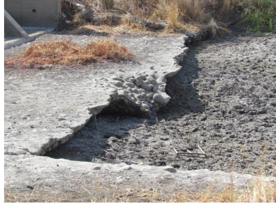
Looking at minor revetment erosion on downstream side of structure. (2015)
