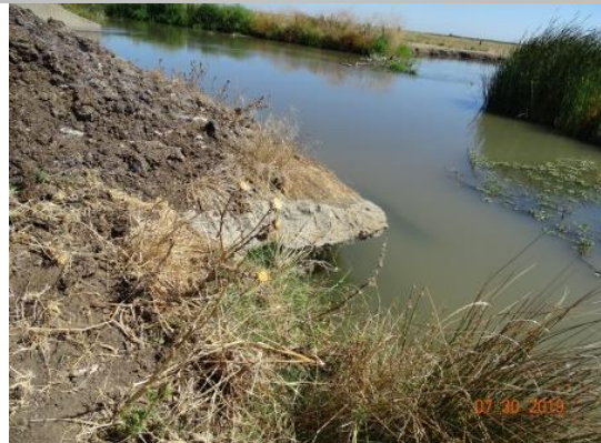
View of erosion at left bank on the upstream side of the structure. (2019)
