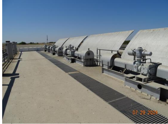
View of the electric gate operators. (2024)
