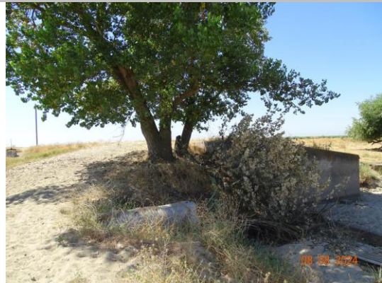
View of the unauthorized pipes through the unauthorized earthen dam. (2024)
