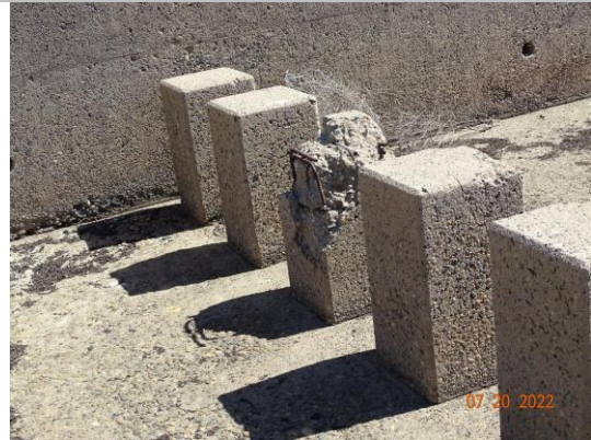
Dissipator near right wing wall is damaged. (2022)
