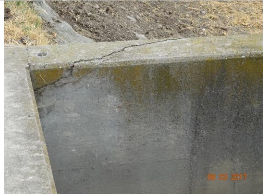
Cracking on left wing wall. (2017)
