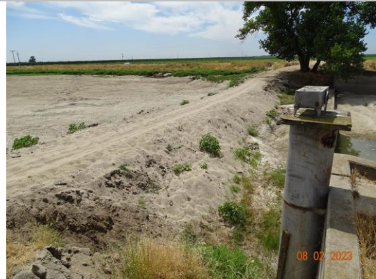
View along unauthorized sand dam from the right bank. (2023)
