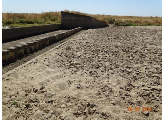
Downstream view of revetment, mostly obscured by sedimentation. (2024)
