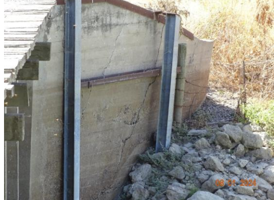
Looking at crack on left wing wall on downstream side of structure. (2024)
