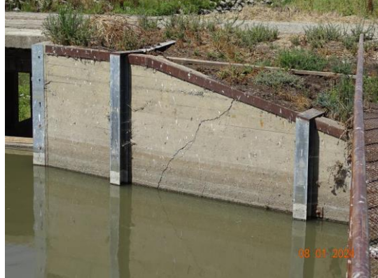
Cracking on the right headwall of the structure. (2024)
