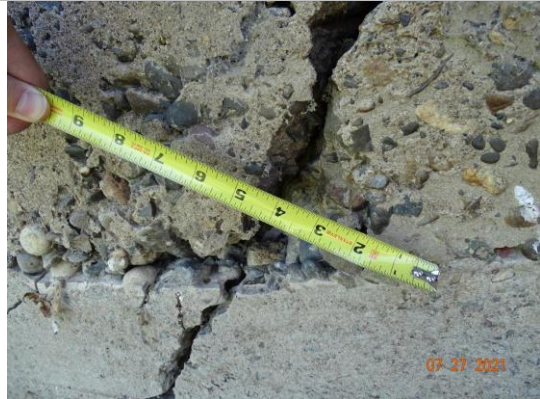
Measurement of crack at the widest section on left downstream wing wall. (2021)
