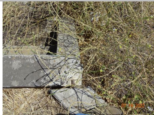
View of cracking at the joint on the left inlet side. (2022)
