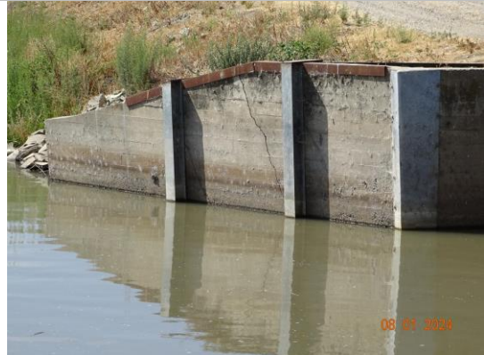
Cracking on the left headwall of the structure. (2024)
