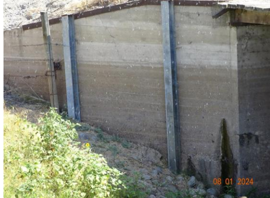
Looking at small crack on right wing wall on downstream side of structure. (2024)
