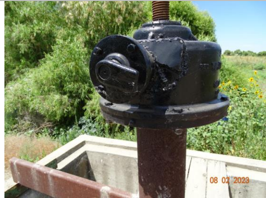
View of the broken crank arm. (2023)
