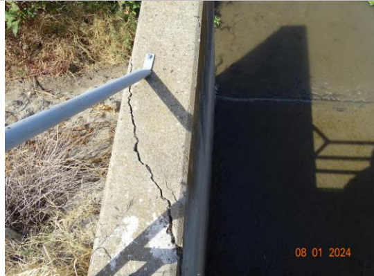
View of crack on the left wing wall. (2024)
