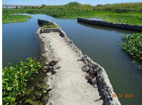
Damage to the left wall of the structure. (2024)
