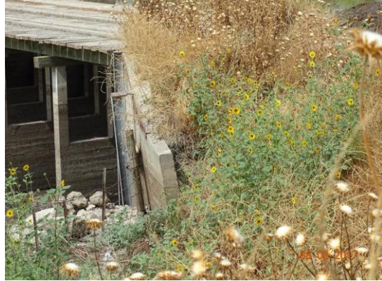
Left wing wall tilting with braces in place. (2017)
