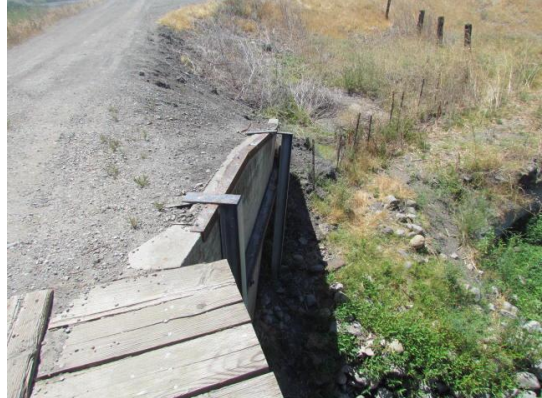
Looking at brace on left wing wall on downstream side of structure. (2012)
