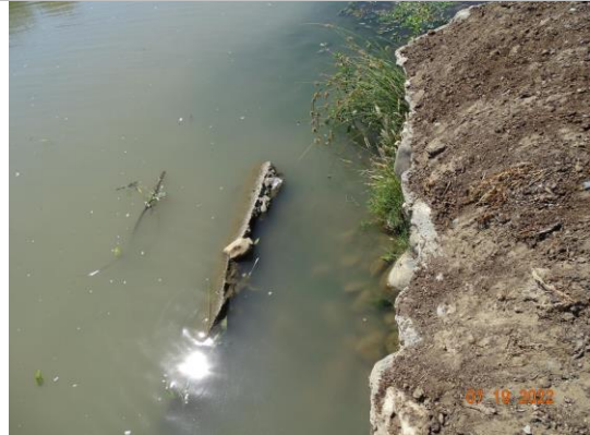
Piece of concrete broken off from the left upstream bank. (2022)
