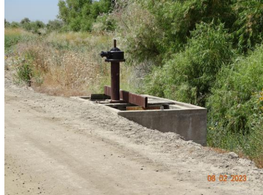
View of manual gate operator at the levee crown. (2023)
