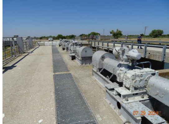
View of electric gate operators. (2024)
