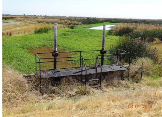
View of manual gate controls. (2024)
