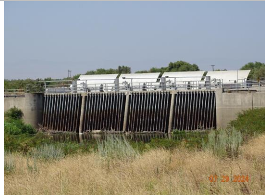
View of trash racks. (2024)
