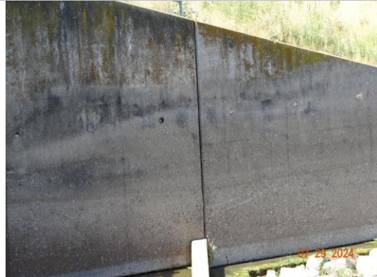
Deterioration of the left downstream wing wall joint. (2024)
