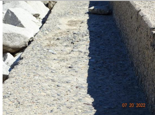
Minor spalling on lip just upstream of the revetment. (2022)
