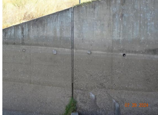
Monolith joint deterioration on the right downstream wing wall. (2024)
