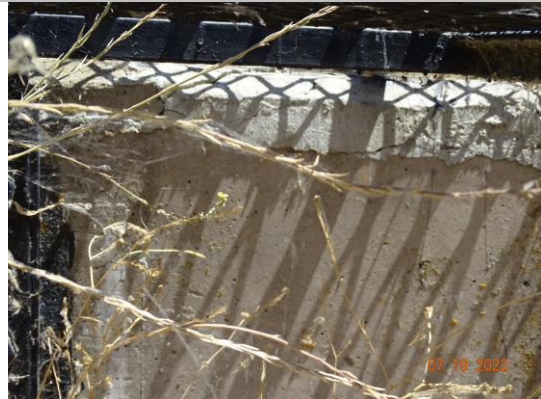
Another view of the cracking on the headwall. (2022)
