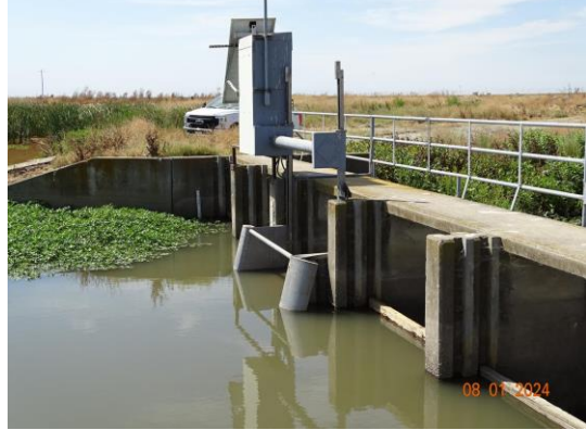
View of the electric gate operator on the upstream side of the structure. (2024)
