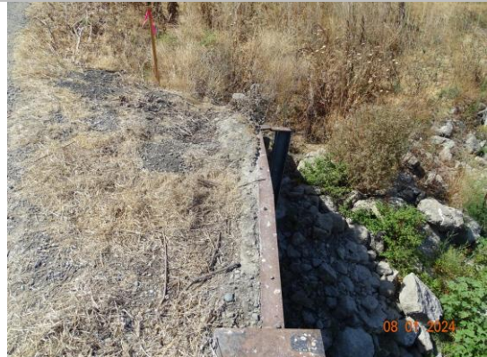
Looking at brace on left wing wall on downstream side of structure. (2024)
