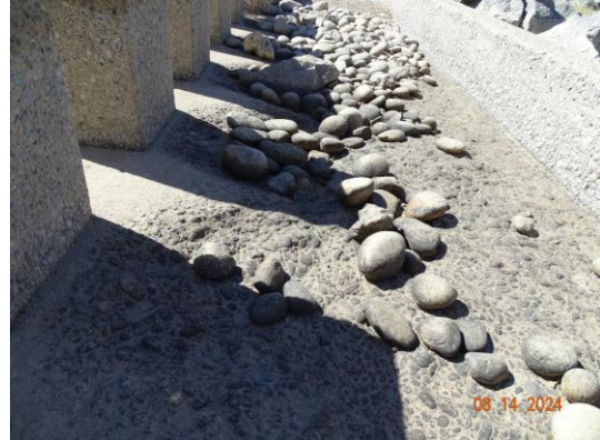
Scour along the base concrete downstream of the dissipators. (2024)
