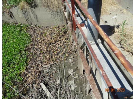
Inlet gates buried under sedimentation. (2023)
