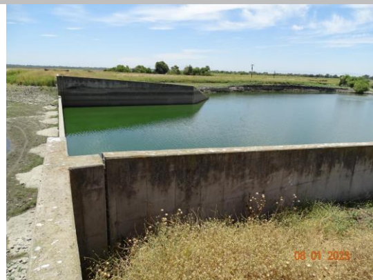
View of right headwall joint deterioration. (2023)
