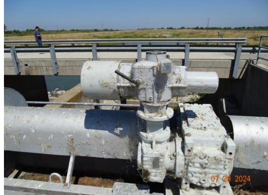
Representative view of electric gate operator. (2024)
