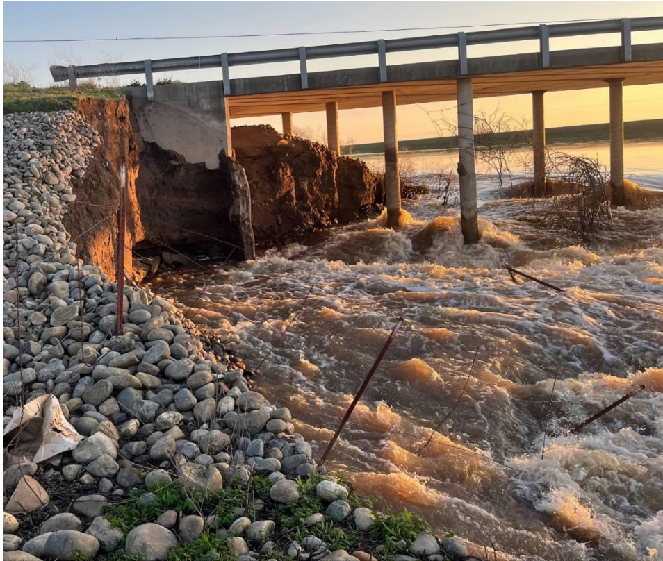
Figure 5-23. Avenue 18 1/2 Bank Erosion
