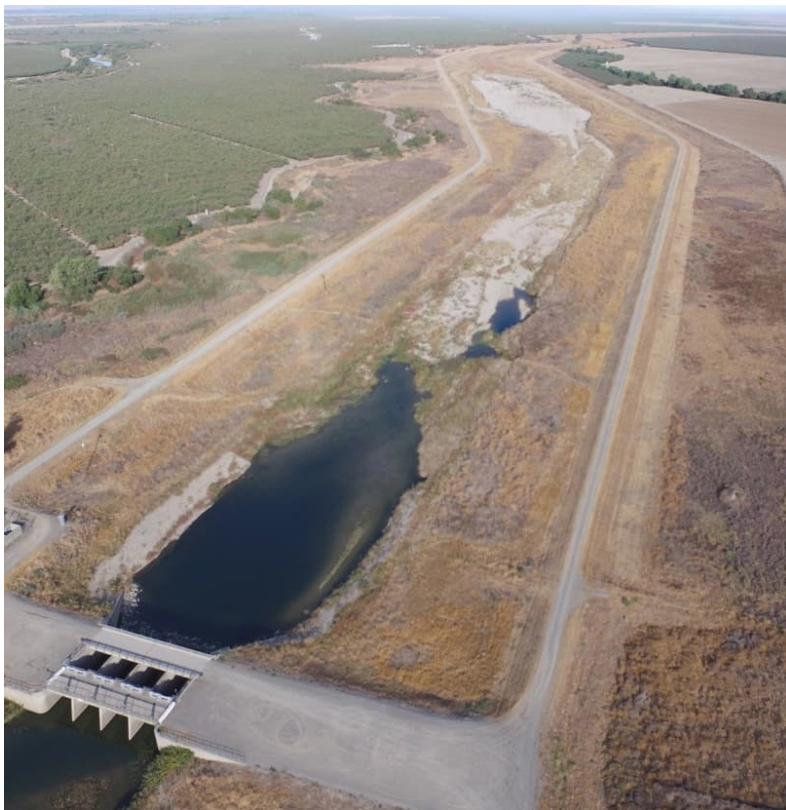
Figure 5-18. Sedimentation in Chowchilla Bypass Downstream of the Chowchilla Canal Bypass Control Structure
