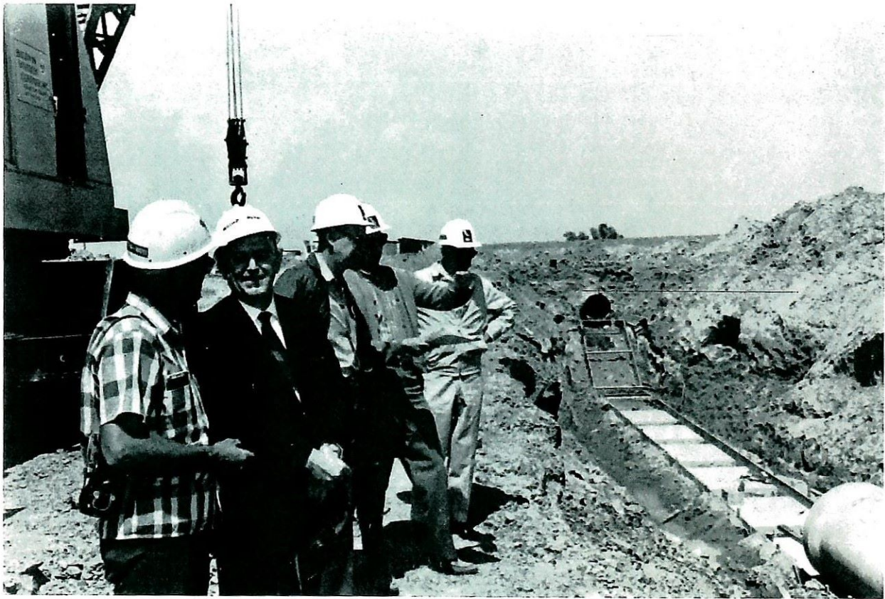
Inspector Pat Dudley; Wm. E. Warne, Director; H. G. Dewey, Assistant Chief Engineer; E. M. McClung, Aqueduct Design Section; and C. H. Carter, Chief, Construction Branch; inspect the East Side Canal Siphon construction.
